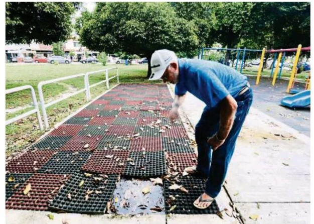
Ravinder showing the poorly installed playground mats at Jalan SS4D/6 in Petaling Jaya. The mats have come loose, allowing water to puddle.
